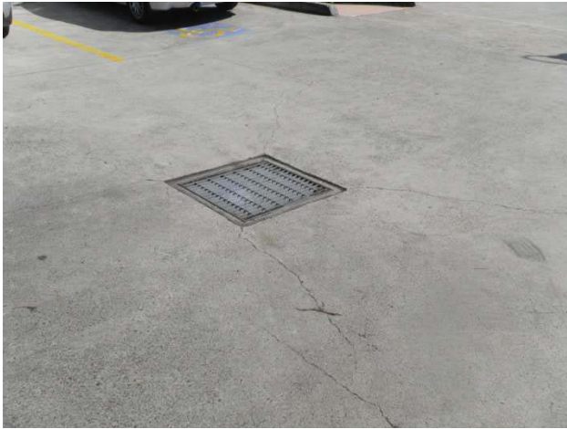
5. Minor cracking around stormwater drains (facing north).
